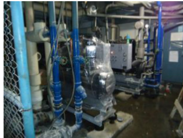
▲ 改善後：新型高效率冰水主機 After improvement: the latest high-efficiency eco chiller
