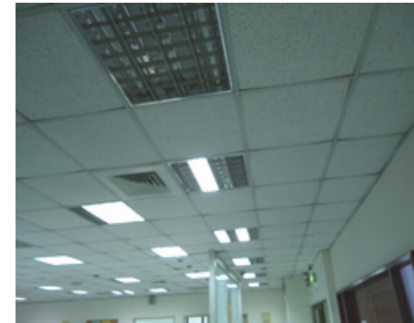
▲ 改善前：T8 燈管 Before improvement: T8 light
