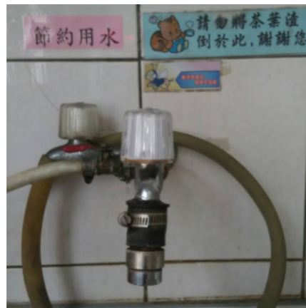
▲ 省水水龍頭 Control valves at faucet
